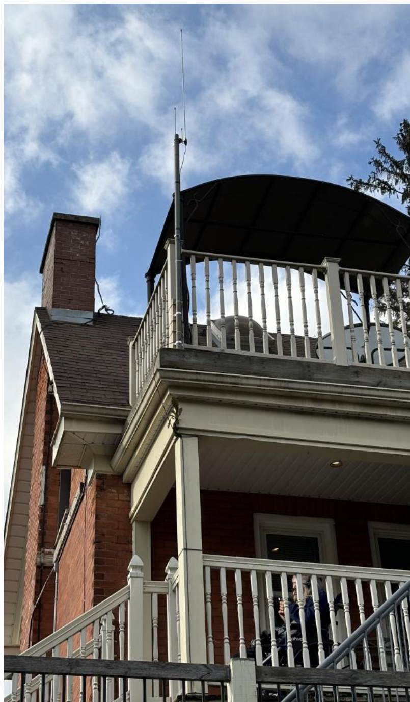
Ted VE3TRQ, Paul VA3PDC, and Tony VE3DWI helped to install the J-pole for Jim VE3JLC who is on the lower deck.
